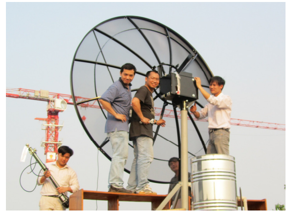
Installation of the SRT : Diep, Dong and INST friends giving a hand
